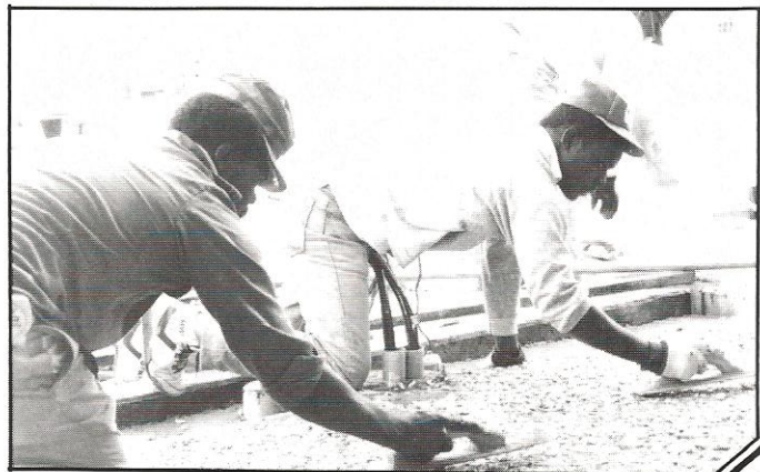
The construction workers crunch the oyster shells into place in the wet cement on a cool April afternoon.
