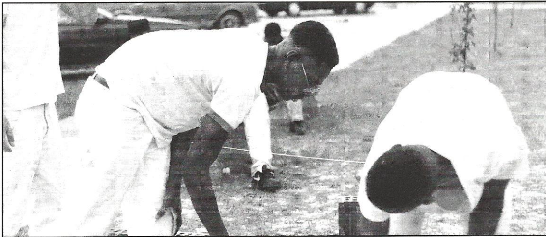
Senior Telly Lewis trowels the mortar between the bricks for the seating project. This was Telly's second year at the Vocational School.
